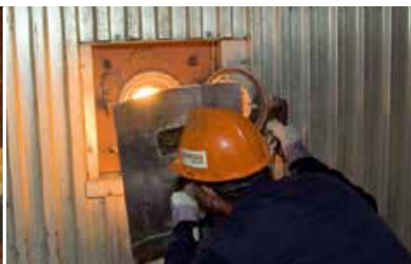
Operator checking fire during biomass test burn.
